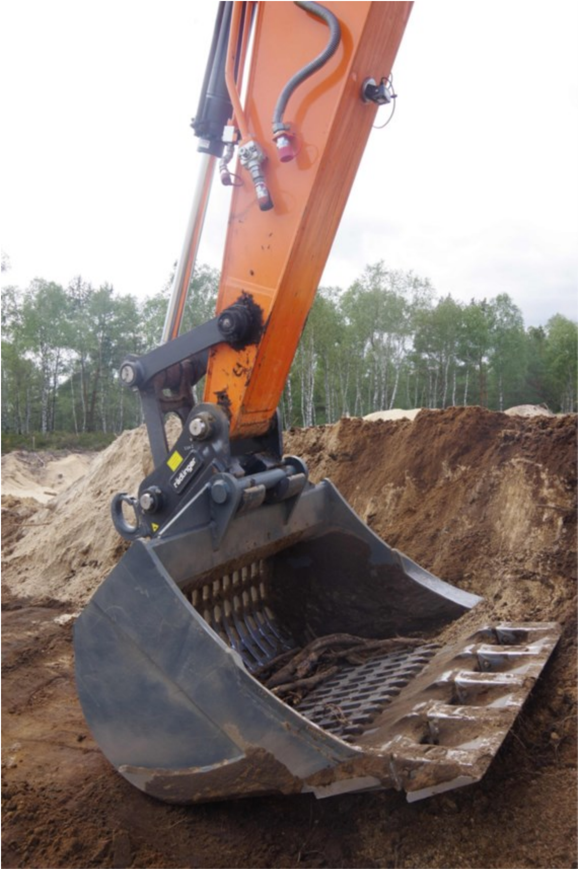
Figure 17: Screening bucket in operation. One of the monitoring cameras can be seen on the arm of the excavator.
