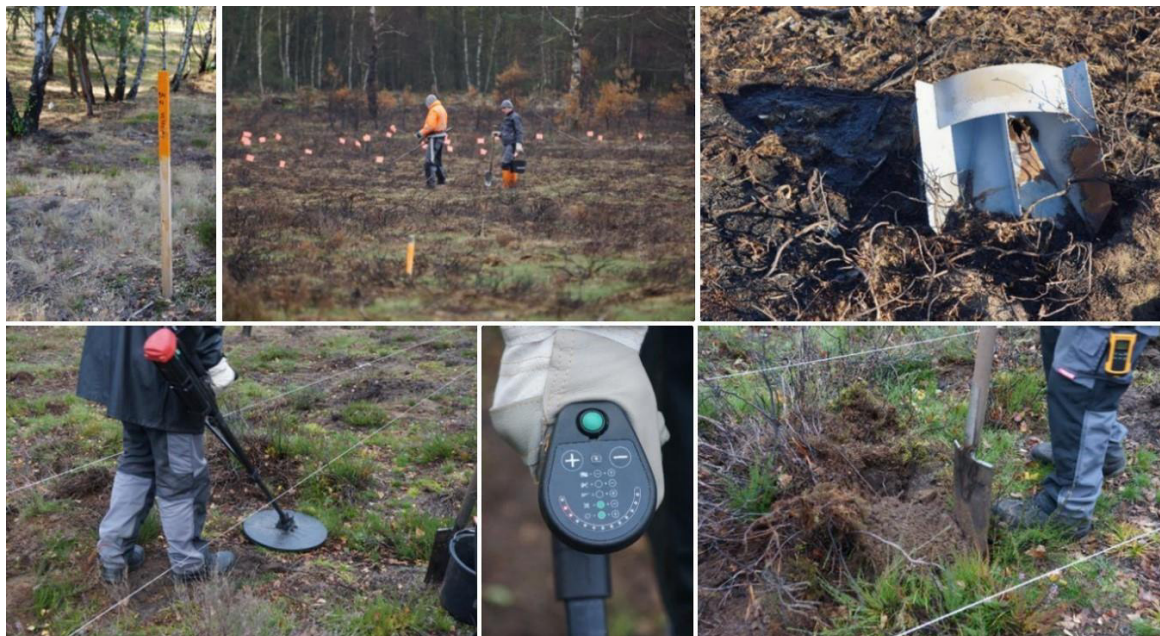
Figure 15: Elements of clearance work: (top row, left to right) plots staked out; anomalies flagged up; a find on the surface; (bottom row) operating the Minelab F-3 UXO detector and digging down towards anomalies
